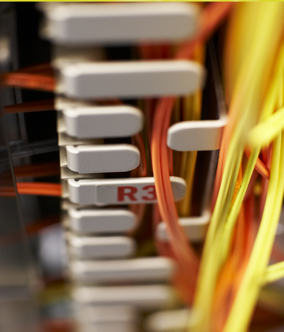
Fiber optic lines have revolutionized telecommunications.
